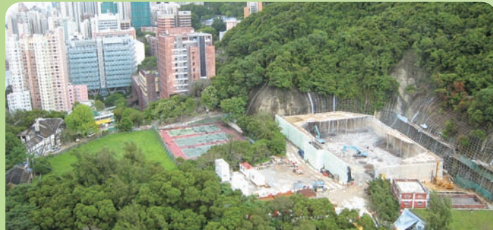
For the Centennial Campus to be developed, the water storage facilities on the site were repositioned in a rock cavern, which was an innovative, environmentally friendly, and first-of-its-kind such solution in Hong Kong. (photo taken in 2007)
