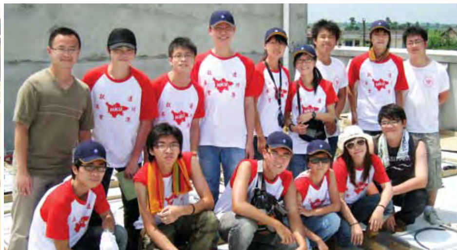
Cindy Cheung (back fourth from right), together with other HKU students, helped to re-build an earthquake-damaged school in Sichuan.
