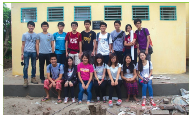
All participated students and the lavatory they helped construct in the past 7 weeks
